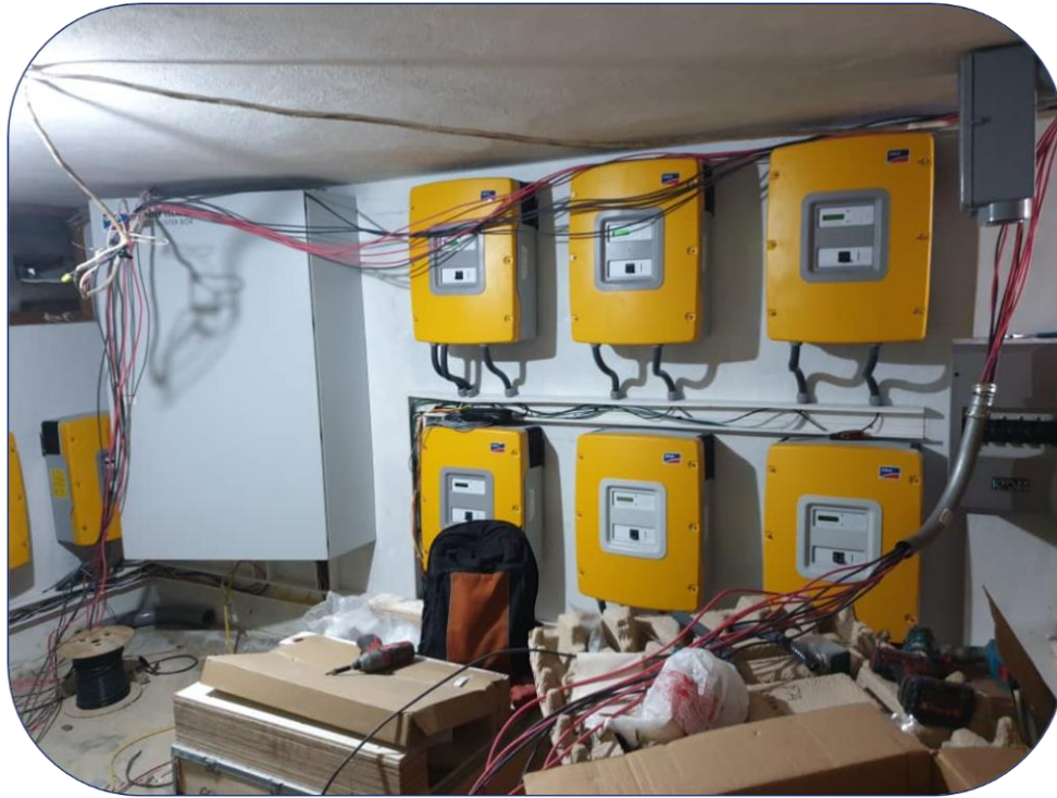
Panels and transformers for the solar system
