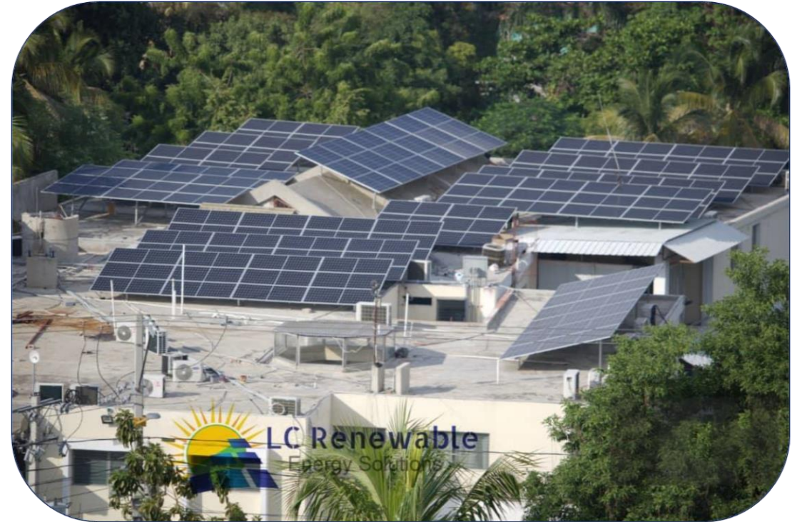
Solar panels on the roof of Hope Hospital
